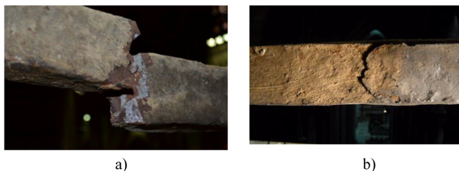
Fig. 3.6. Documentation of iron tie failures: (a) Failure of the iron tie (6th bay T 2-3) [12], (b) Crack in the iron tie (3rd bay, T 2-3) [12].
